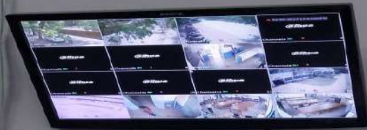
CCTV Surveillance (Girls Hostel)
